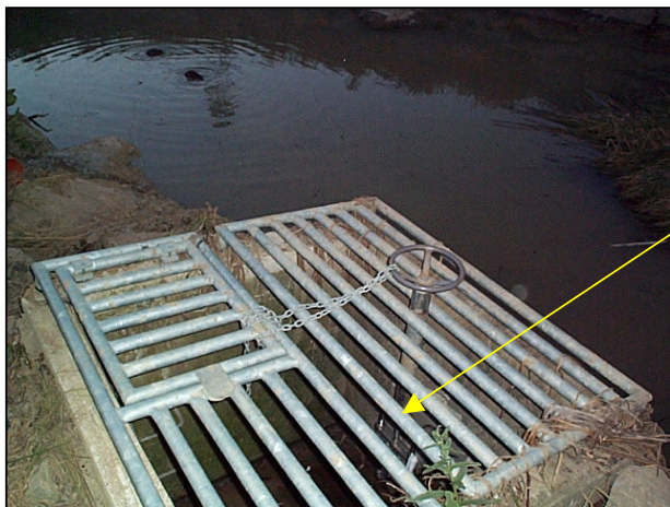
Figure 1.0 Primary drain point with Tyco Keystone Knifegate valve and “external” manual operation.
