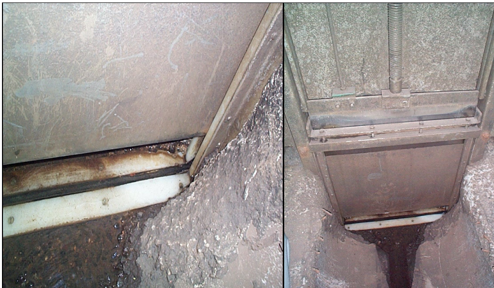
Figure 1.0 Close up and overview of old “penstock” style system
